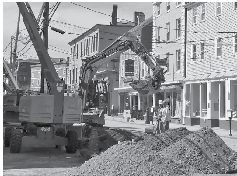
What's the matter, Bunky? Having trouble finding RiverRun Bookstore? Look closer—it's right in the middle of the photo, under the bucket of that excavator. Despite the commotion on Daniel Street, this weekend will be a great time to stop by. April is the store's 20th Anniversary Month! Tom and the rest of the crew are celebrating from Friday the 8th through Sunday the 10th. Everything in the store will be priced 20 percent off.
