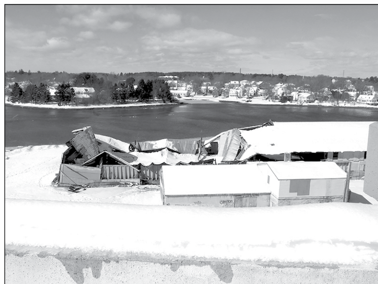
The wholesale firing of the nation's entire cadre of Federal Road Salt Barn Inspectors has led to a predictable result—and a prompt one at that. The storage facility whose wreckage is seen here has stood on this spot since the Mayoral administration of Eileen Foley, at the least, and may even date back to the administration of her mother, Mary Ellen Carey Dondoro.
