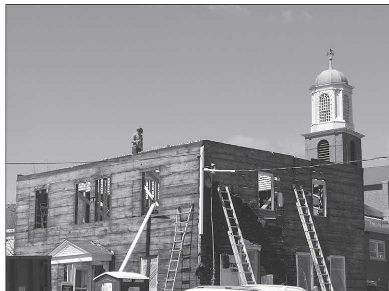
The steeple of St. John's—and the Historical District Commission—watch over the renovation of this Daniel Street duplex. Dormers are coming.
